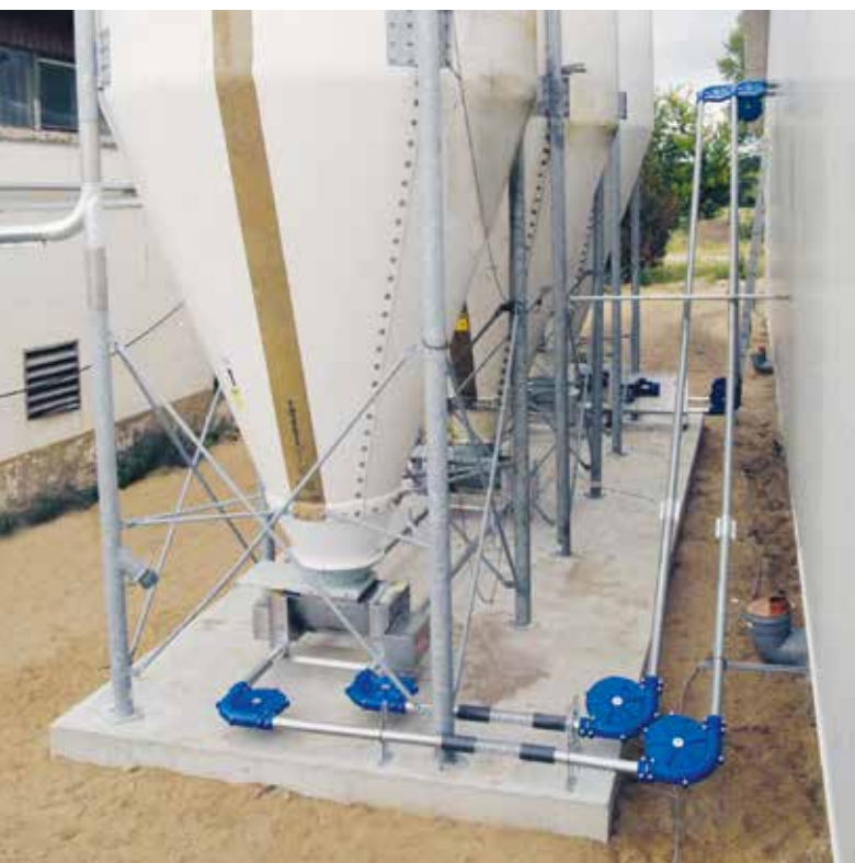
Outdoor silos for dry feeding
