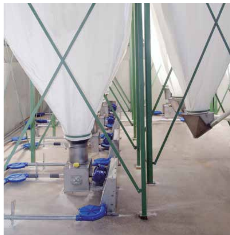
Indoor silos for dry feeding
